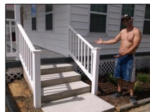
Completed porch stairs and the owner of Hammertime Home Improvement, Mark Hiteshew.
